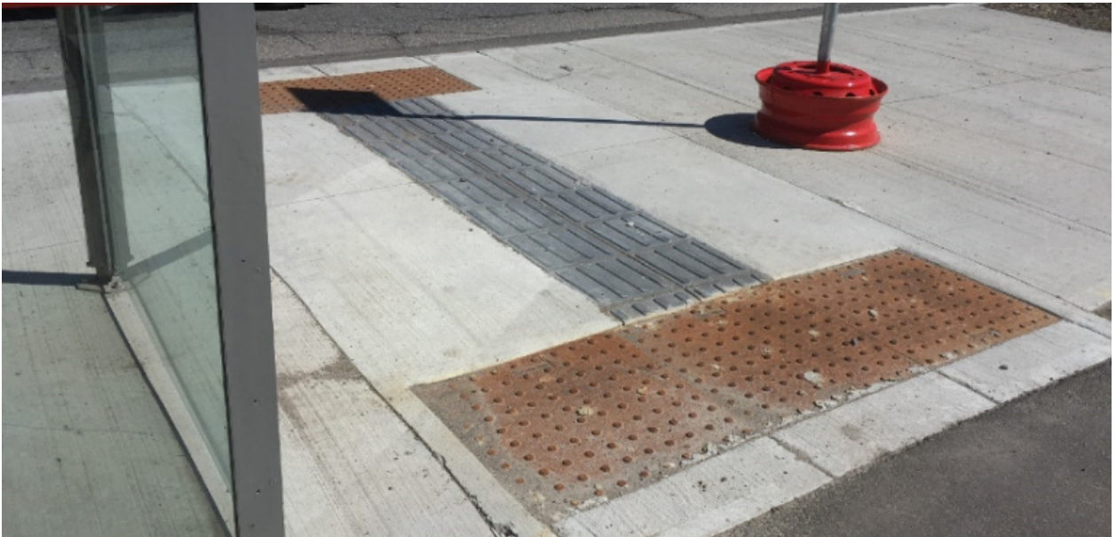
A guidance TWSI in grey used to guide pedestrians between a bus stop (left) and a cycle track crossing (right). Red attention TWSI's are used to identify hazards at each end. Ottawa, ON
