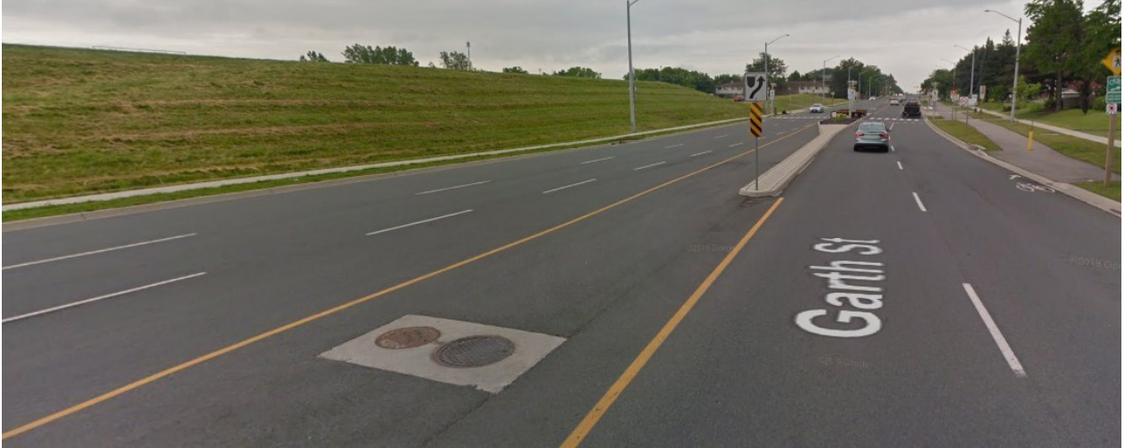
Maintenance holes positioned outside the wheel path of motor vehicles and bicycles on Garth St. in Hamilton. Source: Google Maps
