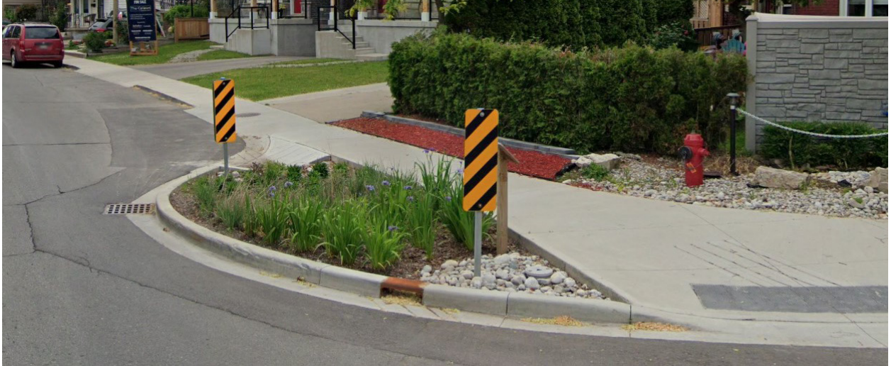
A Rain Garden Traffic Calming Bump-out installed at the intersection of Bay Street North and Simcoe Street in Hamilton. Source: Google Maps
